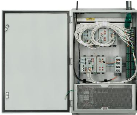
Figure 3. Integrated Network Zone systems from Panduit can offer 75% reduction in time to deploy. 1
